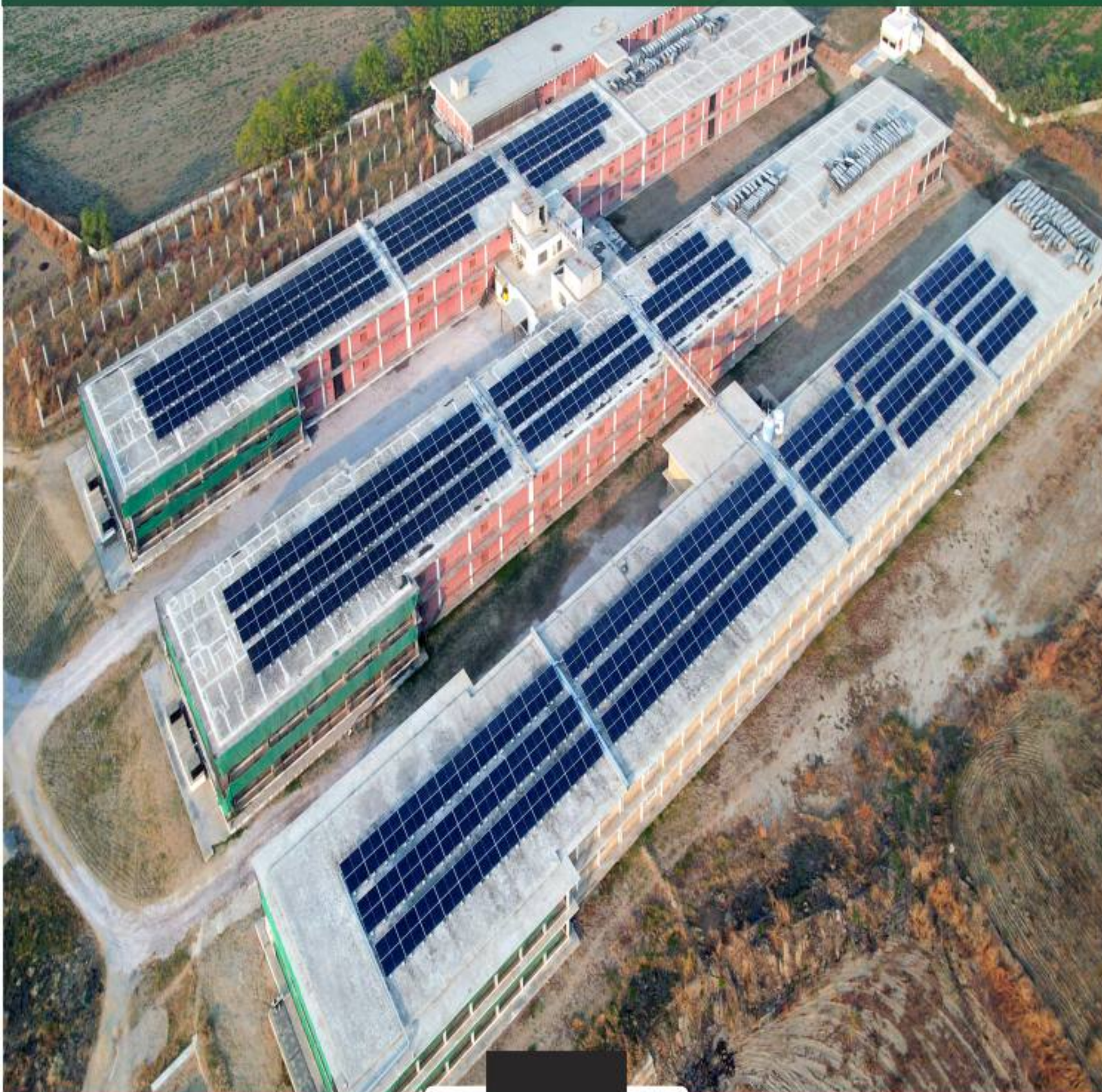
140 kW Grid-Tied Solar Power Plant at Awan Cold Storage, Peshawar
