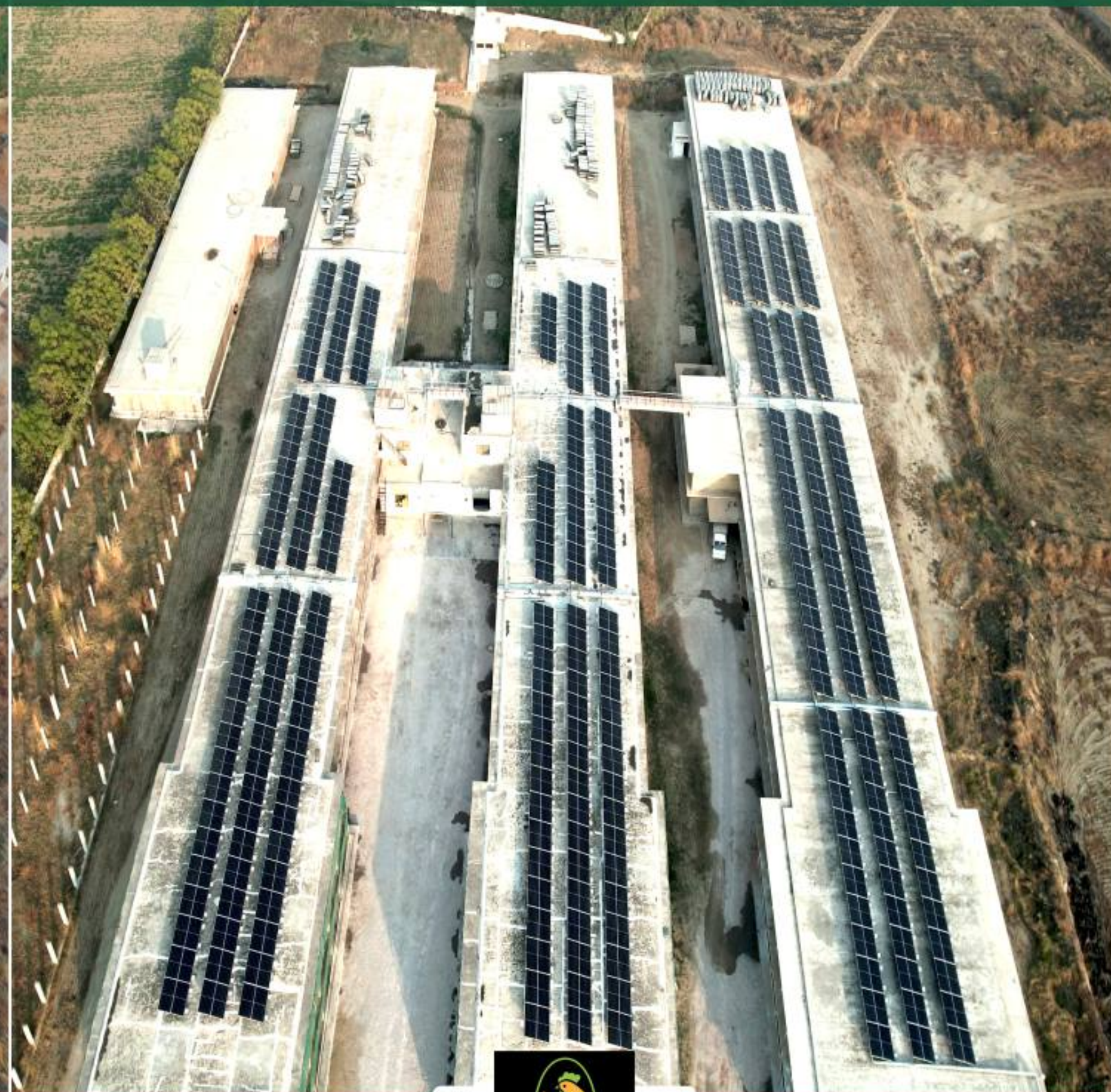
1.42 MW Grid-Tied Solar Power Plant at Al Abbas Poultry, Attock
